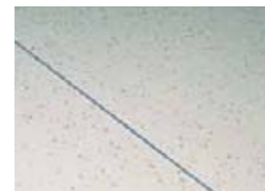
1 Grind joints to a depth of around 1.5 mm according to the thickness of the product
